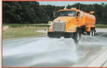
2,000 Gallon Water Tank
